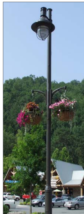
The new LED streetlights installed in Cherokee will result in annual savings of $23,000.
